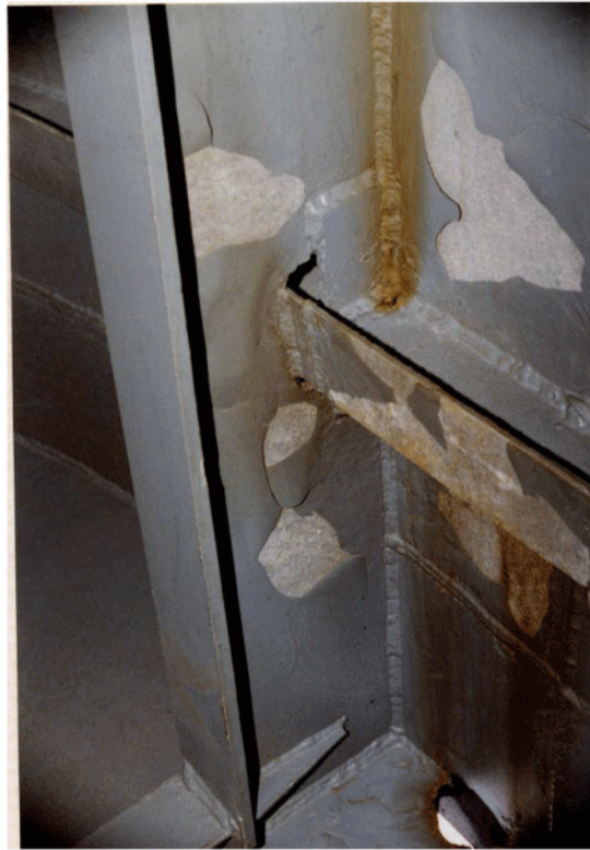
Disbonded Coating on Aluminum Structure
