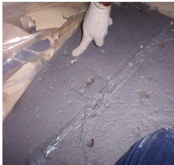
Deeply pitted tank bottom shell plate
