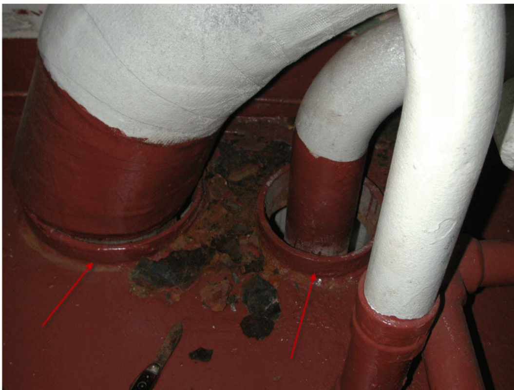
B. Non-Tight Reinforcing Ring at Deck Piping Penetration
