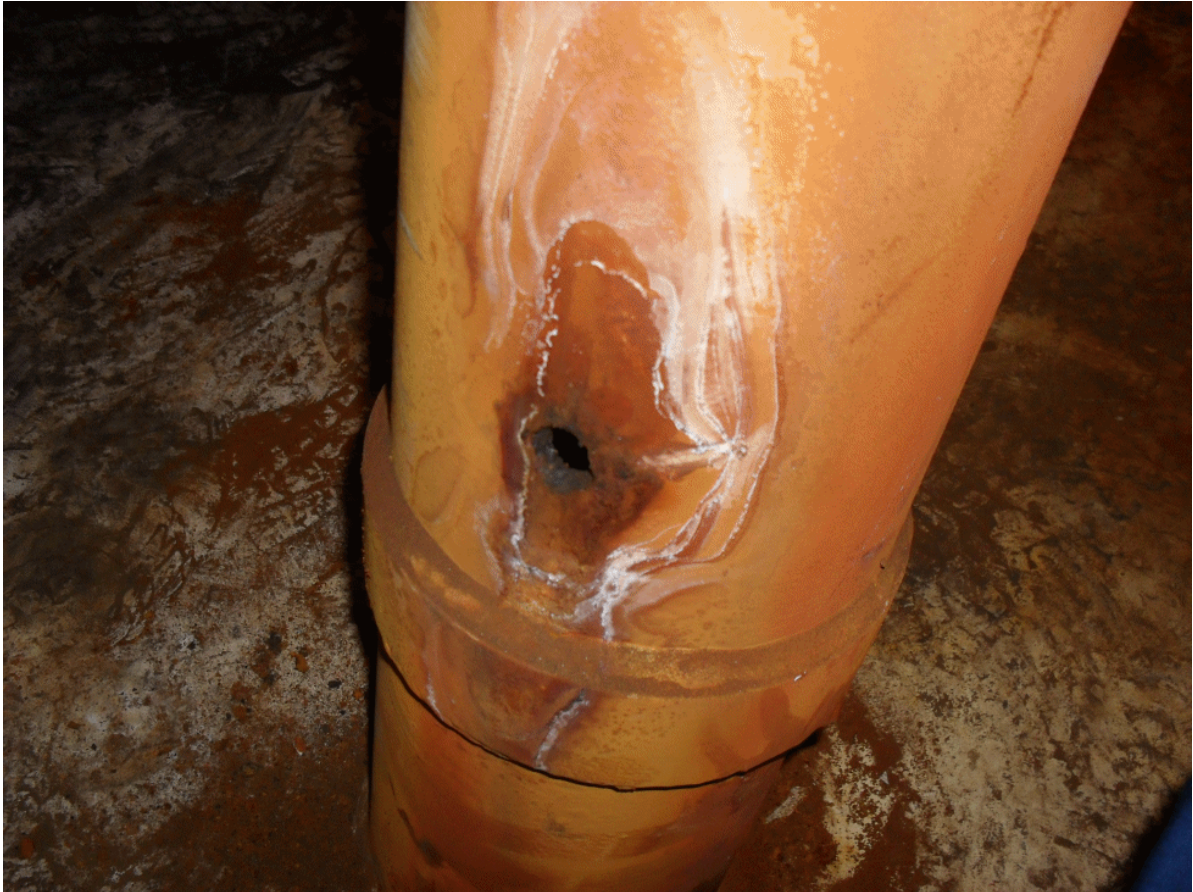
Figure 4-8 Corroded And Holed Degaussing System Conduit In A Tank
