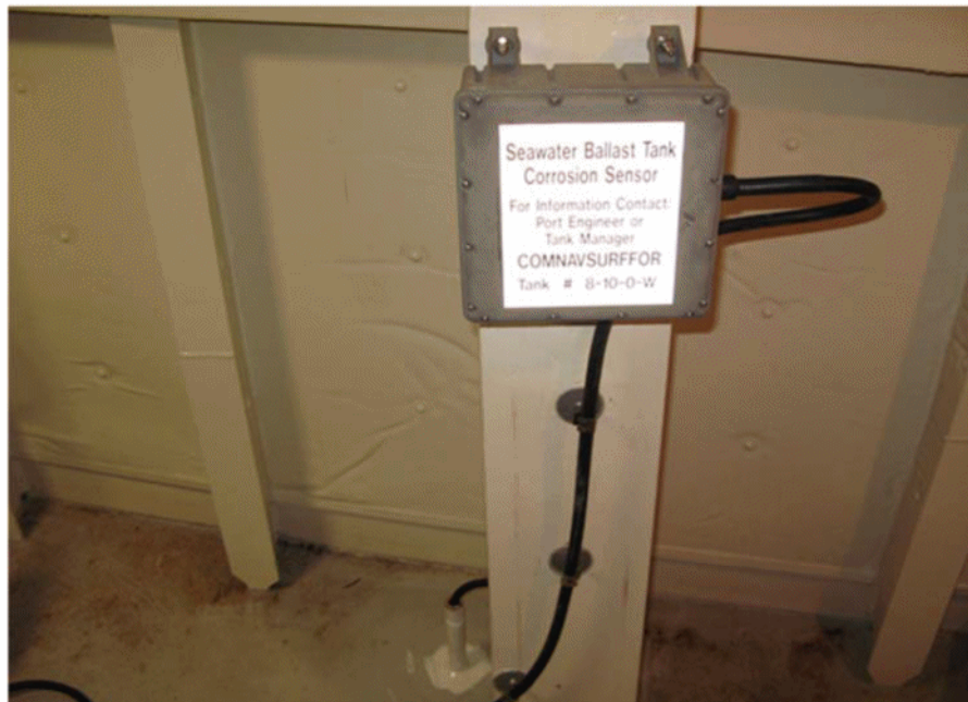
Figure 3-2 Typical TMS Installation In Tank (Top) and Data Logger (Bottom)
