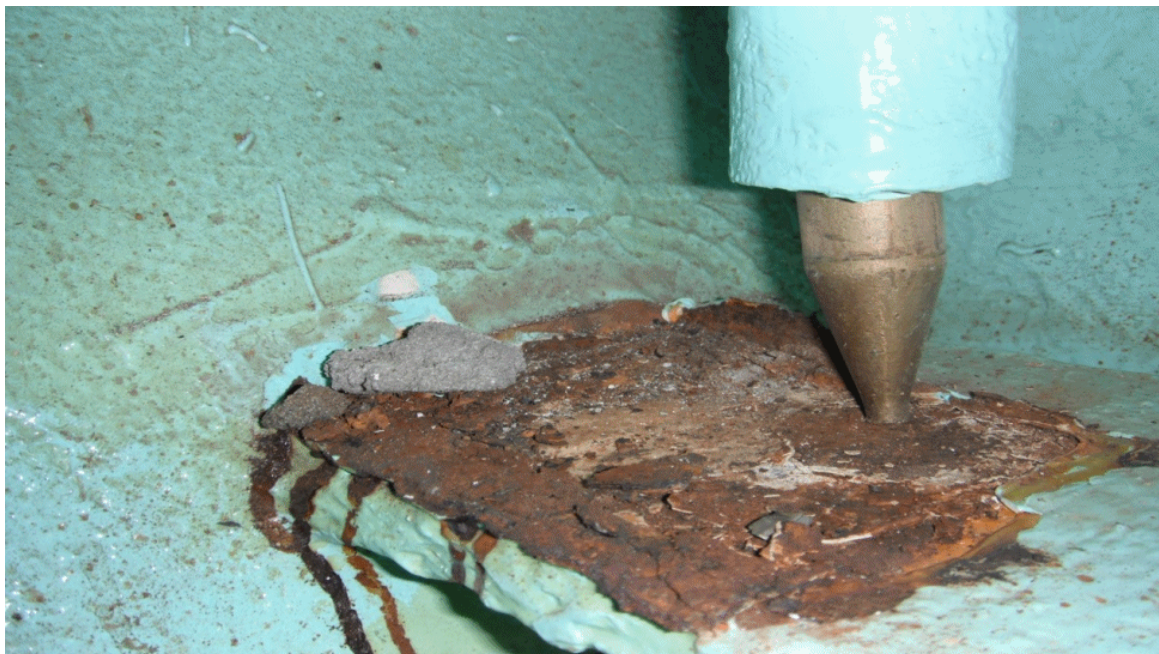
Figure 4-7 Coating Damage and Corrosion of Sounding Tube Bob Striker Plate
