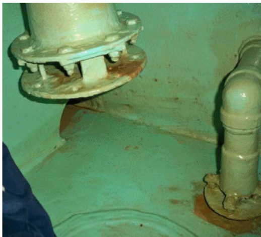
A. Waster Installed On Pipe
