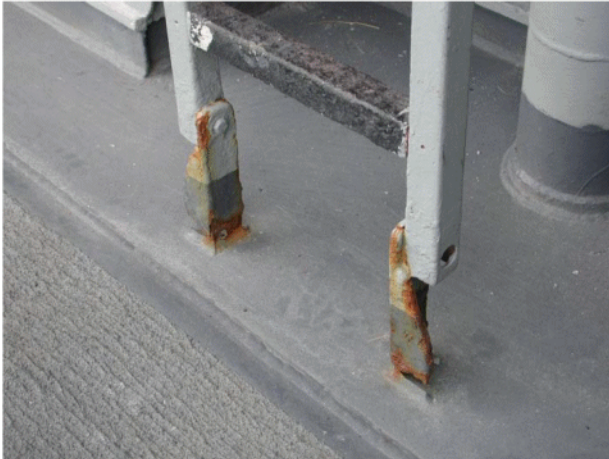
GRP Ladder and Steel Supports
