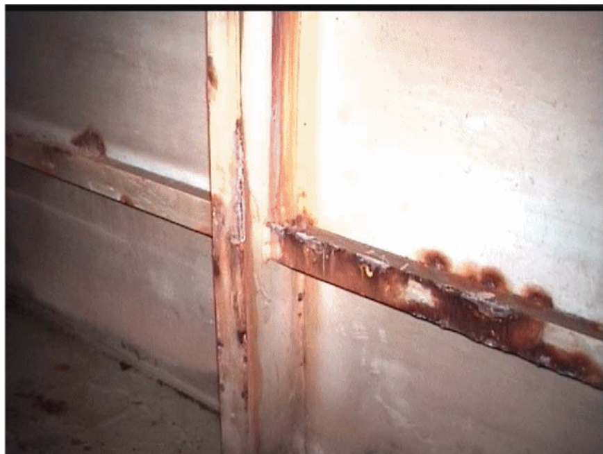
B. Coating failure initiated at stiffener edges and welds
