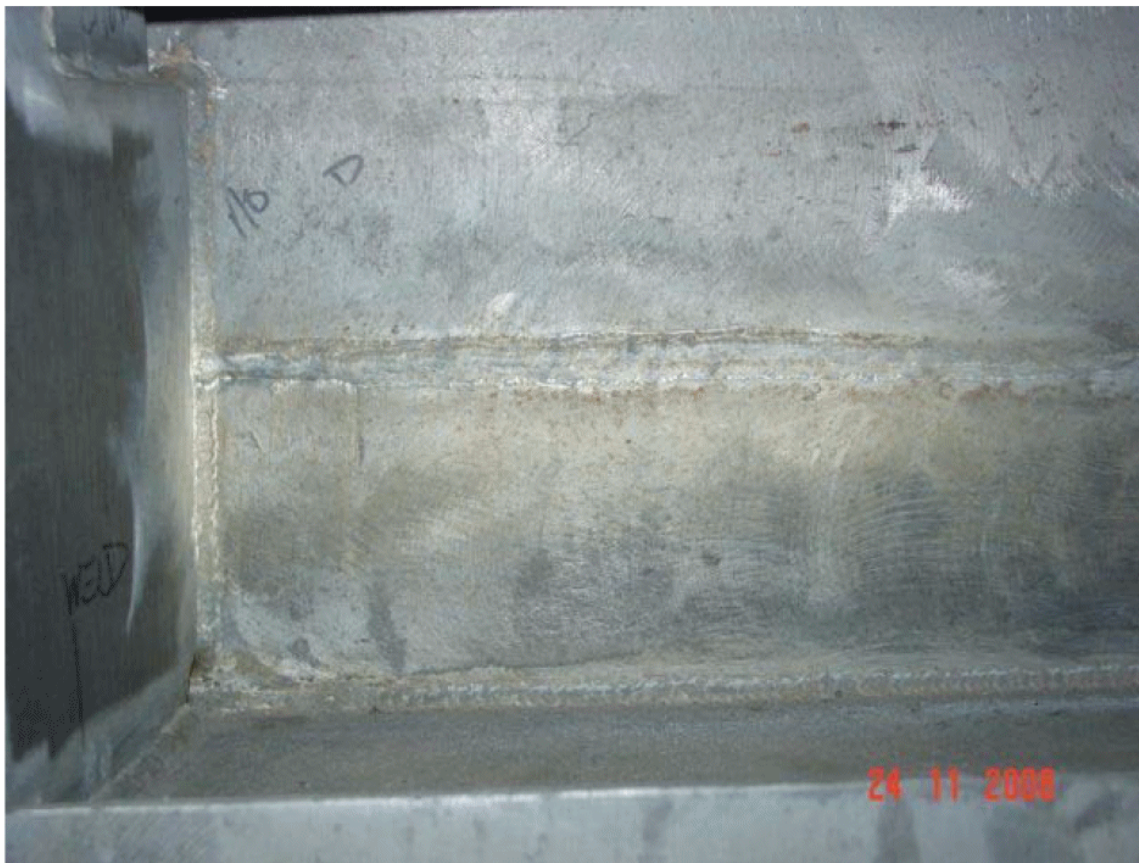
Figure 4-1 Bare Aluminum Water Tank With Acceptable Oxidation
