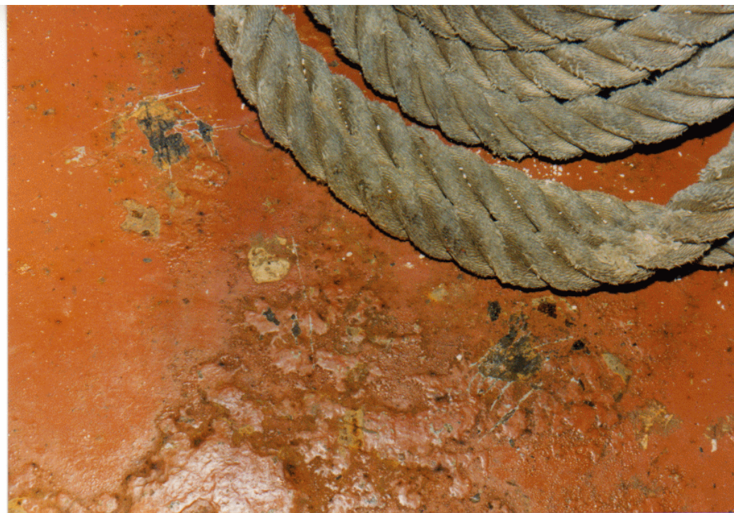
Figure 4-14 Blister-Like Coating Failure Over Rust
