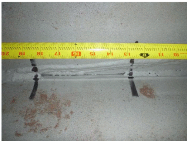
Incomplete Fillet Weld
