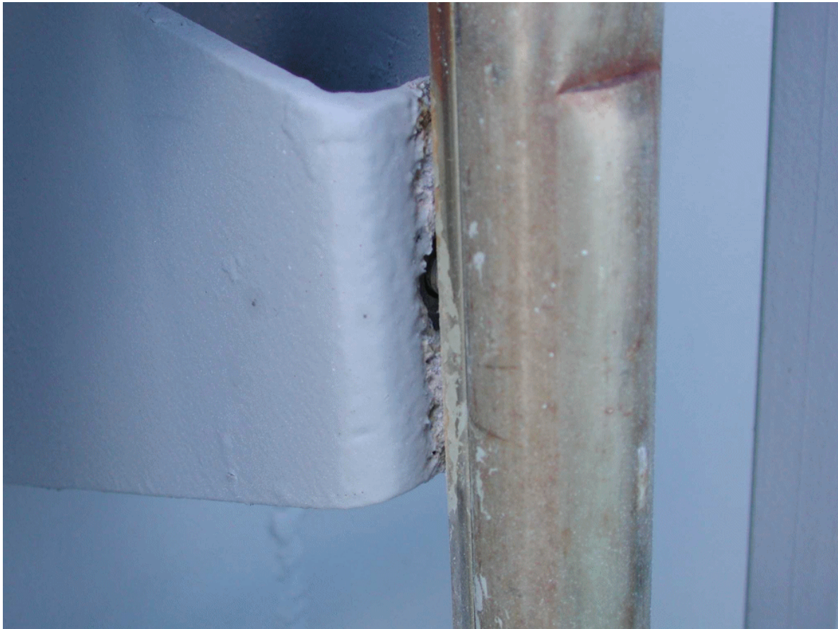
Figure 4-4 Corrosion of Aluminum Support for Stainless Steel Climber Safety Rail
