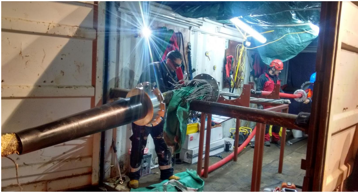
Figure 13. Orbital Marine Power and HV Contractors offshore on a multi-cat vessel cable jointing or “splicing” operations where static cables are permanently connected to the platform cable which supplies power and communications.
