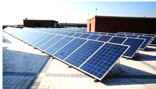
Fig. 3. Roof top solar power PV plant 52)
