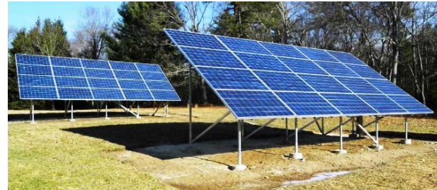
Fig. 2. Ground mounted solar PV 51)
