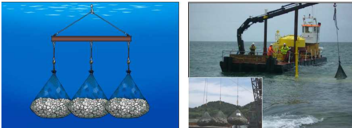
Figure 6 Installation of rock bags in lines using a beam and single units placed with a rope.
