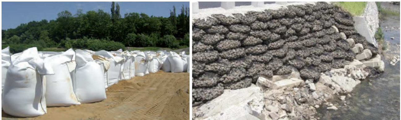
Figure 2 Example of geobags (left) and rock bag protecting a river bank (right) (from the web)
