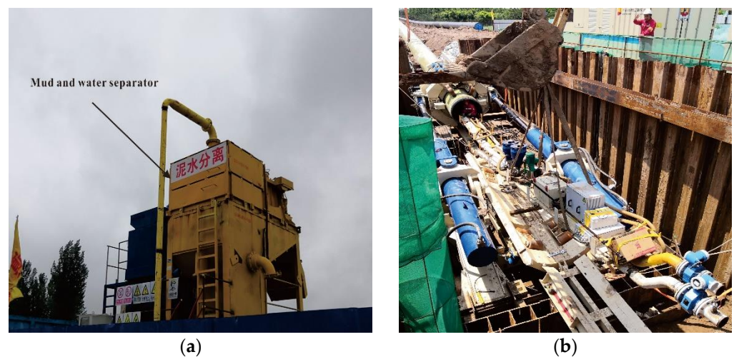
Figure 11. The project mud–water separation equipment and installed pump: (a) mud–water separation equipment; (b) installed pump.
