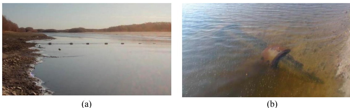
Figure 3. Scours and denudations of the I-st and II-nd lines of the underwater gas pipeline across the Hatasskaya channel: – the position of the inverted siphons above the water surface, b) – line-II is visible through the water.
