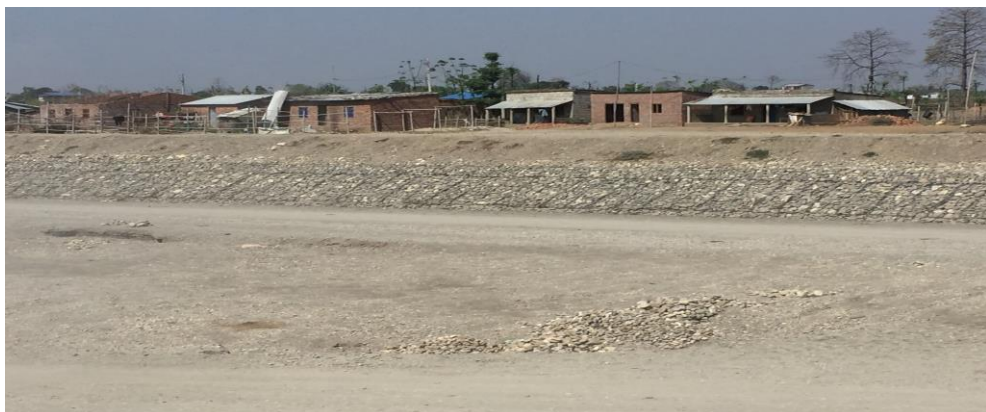
Figure 5. Installed Gabion mattress and launching apron in a bank of the Kayar khola.
