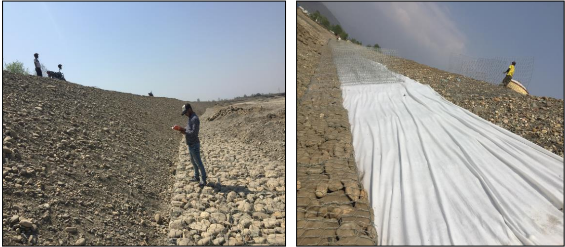
Figure 12. (Left) Foundation preparation on slope and (Right) Installing of geotextile fiber below the gabion mattress on slope area.
