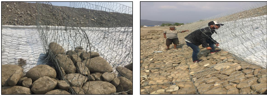
Figure 13. Stone in a gabion mattress (left), and placement of gabion mattress on the geotextile (right).
