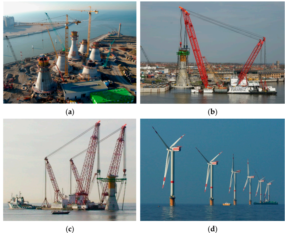
Figure 8. Construction and installation of gravity-based substructures for Thornton Bank wind farm: (a) construction yard by the access channel to the port of Ostend, Belgium, (b) load-out operation, (c) transport and installation and (d) after turbines installation. Credit: C-Power NV, reproduced with permission.
