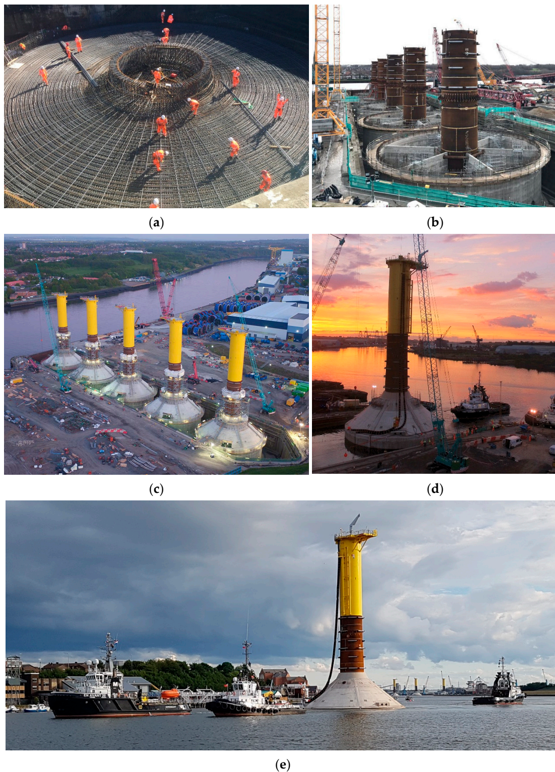
Figure 12. Construction of gravity-based concrete substructures for the Blyth Offshore Demonstrator Project: (a) reinforcement placing, (b,c) construction of the concrete base and steel shaft of the substructures in the dry dock, (d,e) transport of the self-floating substructures using tugboats. Credit: BAM Nuttall, reproduced with permission.
