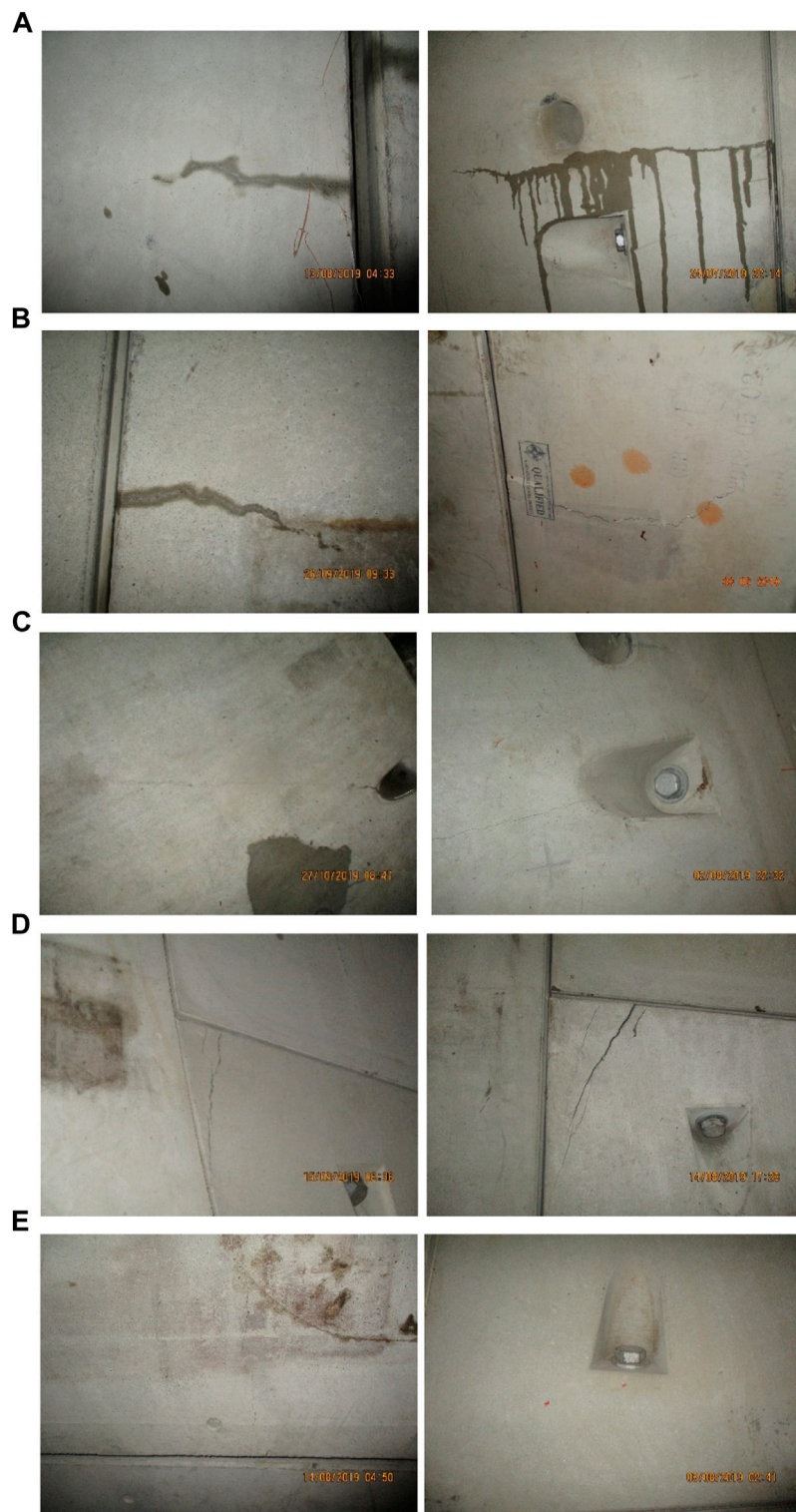
FIGURE 4 Typical cracks: (A) positive crack, (B) backward crack, (C) bolt crack, (D) corner crack, and (E) circumferential crack.
