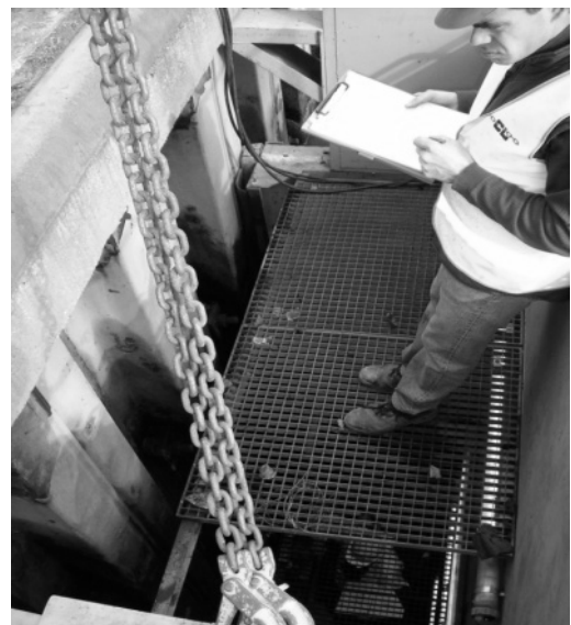
Figure 6. Corrosion inspection of surface condition
