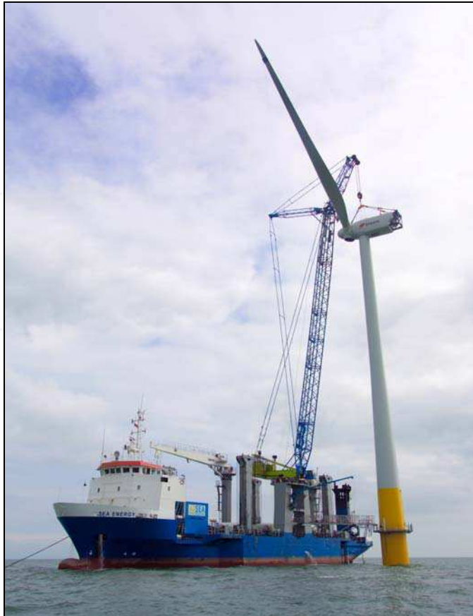
Fig. 22. Wind Turbine being erected with a crane from a special ship at Kentish Flats Offshore Wind Farm, UK (Courtesy: Elsam)
