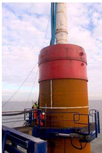
Fig. 8. Menck Pile driving hammer atop a steel pipe pile at Kentish Flats Offshore Wind Farm, UK (Courtesy: Elsam)
