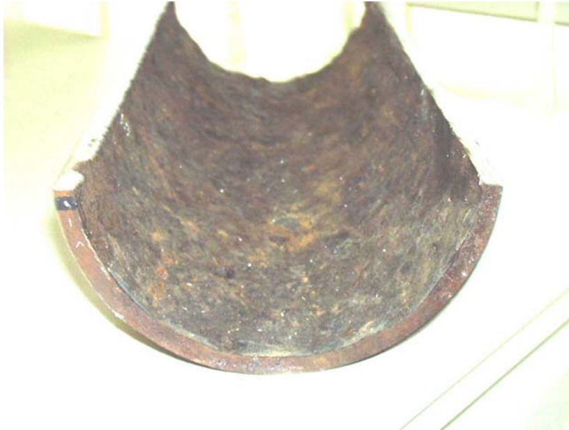
Figure 19a Corroded Pipe Sample
