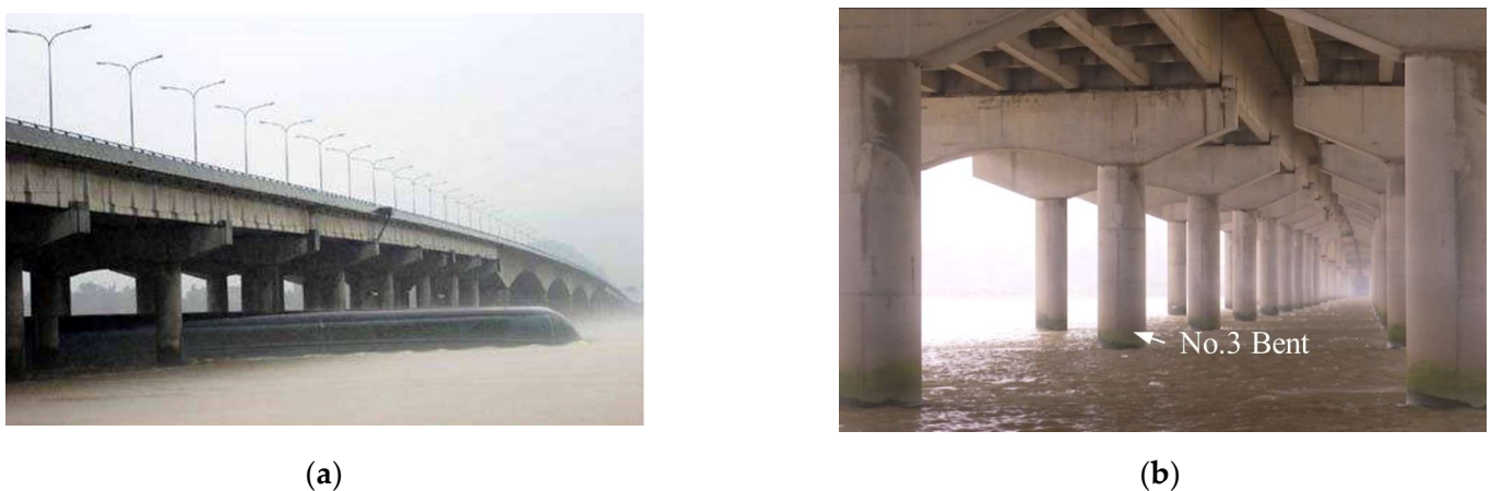
Figure 7. Photos of the Wulong River Highway Bridge: (a) overview of the bridge; (b) the No.3 Bent.
