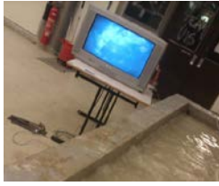
Figure 6: Leaking water detected in similar manner as gas
