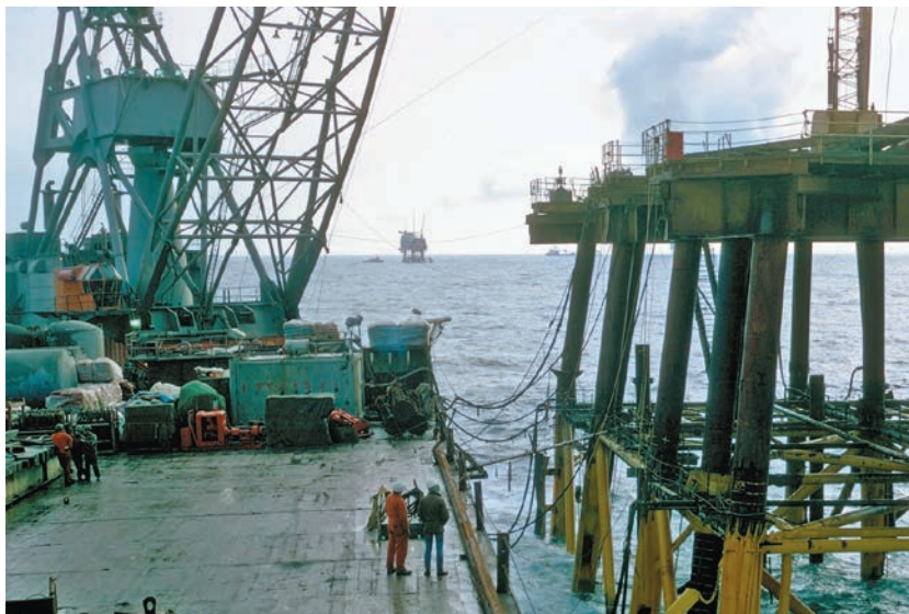
A hectic construction phase. The prefabricated steel platform jackets were shipped out to Ekofisk on barges and piled into place. The divers had to investigate the seabed before a jacket was installed.
