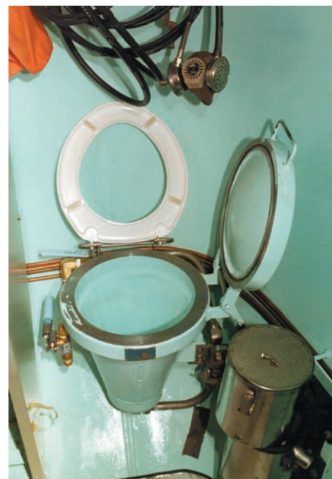
The toilet in a pressure chamber. Photo: Geir Ivar Jørgensen
