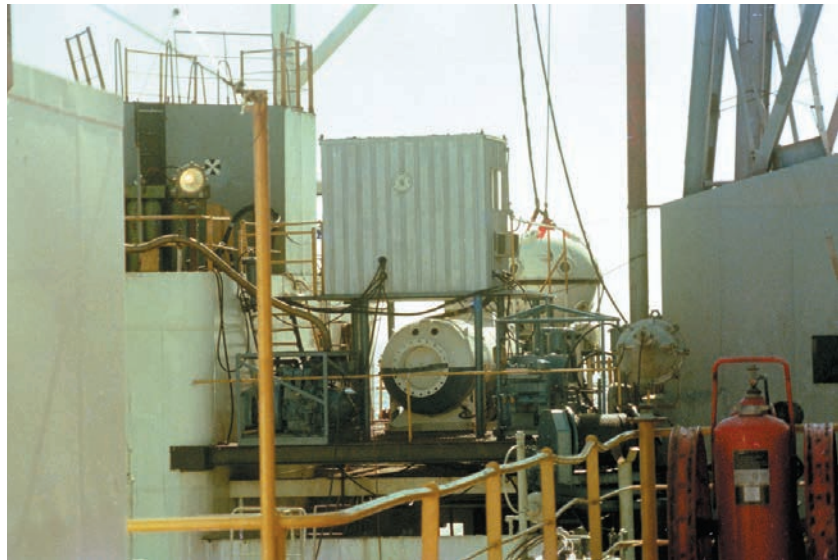
The Ocean Systems bell diving spread, with bell, deck decompression chamber (DDC) and control room, on Gulftide in 1974. Photo: Hans Claesson
