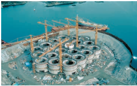
The first stage in building a Condeep GBS at the Norwegian Contractors dry dock in Stavanger. Casting these structures took place in Stavanger, Åndalsnes and Hanøytangen outside Bergen, while the Ekofisk tank's breakwater was cast in the Åls Fjord. Photo: Statoil
