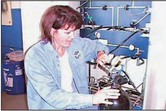
FIGURE 5.28 Air Fill Control Panel With Fill Hoses
