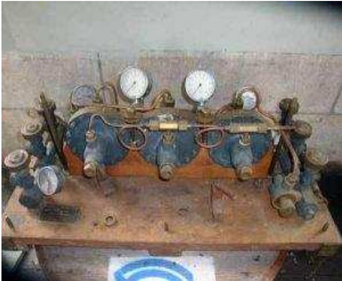
Photo n° 19: Automatic gas control unit (45)
