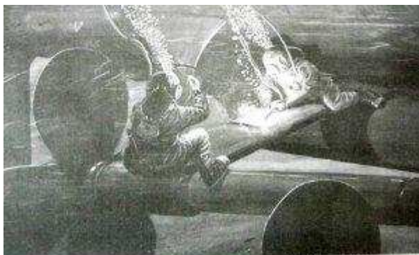
Fig. 14. Removing starboard side propeller shaft of H.M.S. Galena during the Second World War with B.G.C. "Sibyl" (British Gas and Torch system)
