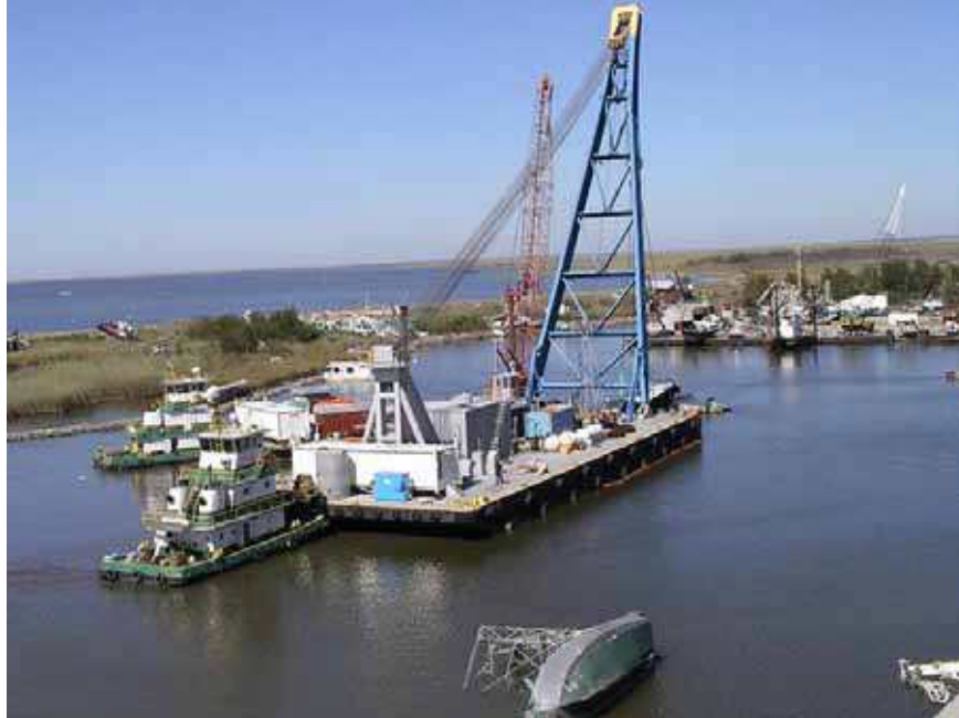
Figure 4-4. T&T's Big T and George T preparing for a lift in Empire, Louisiana.
