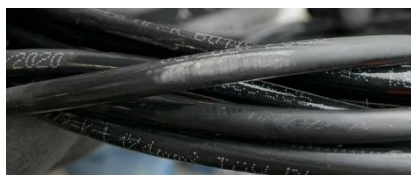
Figure 8: Cable 2 (saltwater tank) showing signs of physical degradation of the insulation layer.
