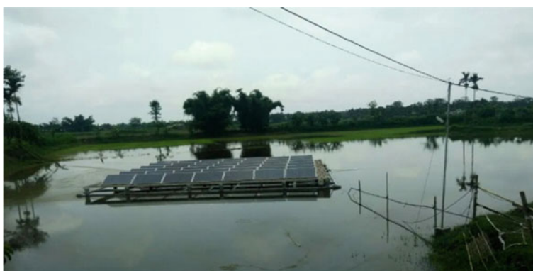
Fig. 6 10.5 KW FPV plant in Assam [12]
