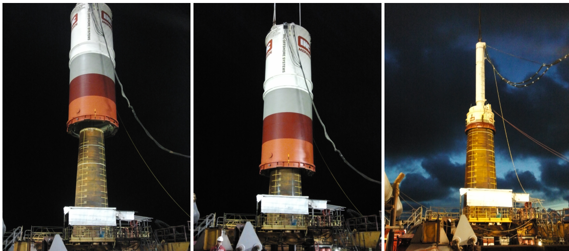
Figure 15. The installation of a 6.5 m pile with the use of a Noise Mitigation Screen (IHC Offshore Systems) at the German offshore wind farm Riffgat in the North Sea. In the left and middle pictures, the NMS is positioned by the crane around the monopile. In the right picture, the hydraulic hammer is positioned at the head of the pile and the NMS is invisible (positioned lower than the deck of the installation vessel). Source: Author's personal archive from the Riffgat Offshore Wind Farm (2012).
