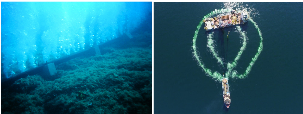
Figure 12. (Left) Air-bubble cloud released by a perforated pile positioned on the seabed. (Right) Double Big Bubble Curtain (DBBC) deployed around the Giant7 floating piling vessel in the Wikinger OWEF, Germany. Source: © Hydrotechnik Lübeck GmbH ( https://www.hydrotechnik-luebeck.de/blog/portfolio-item/0003-borkumwest2-00/ ).
