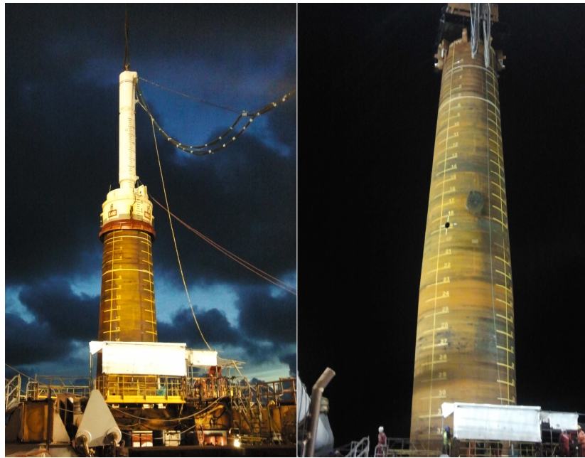
Figure 1. Installation of a pile with an impact hammer (left) and with a vibratory device (right) [19]. Source: Author's personal archive from the Riffgat Offshore Wind Farm (2012).
