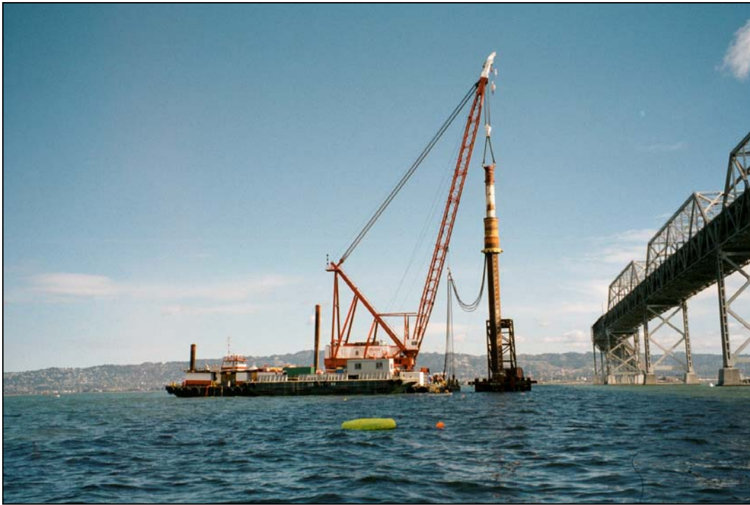
Figure 1-5. PIDP Barge and Large Hammer. (Note: Buoy in the foreground was used to support underwater sound monitoring instruments.)
