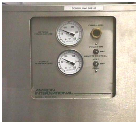
Figure 2-14. Environmental Control System (ECS) Compressor
