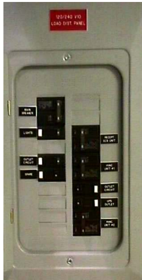
Figure 3-3. Power Distribution Panel (50-amp Main Breaker)
