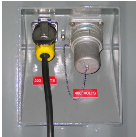
Figure 3-1. Power Receptacle Box
