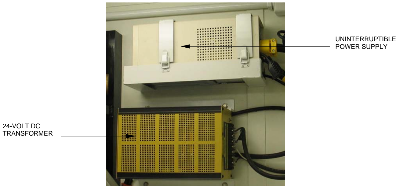
Figure 3-4. Uninterruptible Power Supply and Transformer
