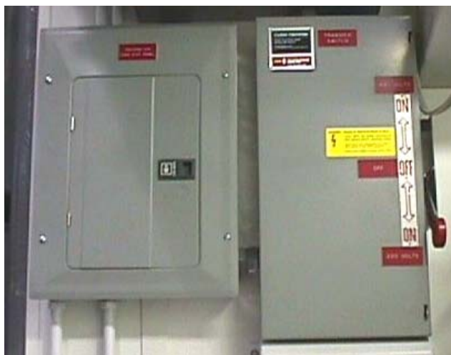
Figure 2-1. Power Distribution Panel (left) and Manual Bus Transfer (MBT) Switch
