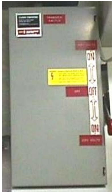
Figure 3-2. Manual Bus Transfer (MBT) Switch
