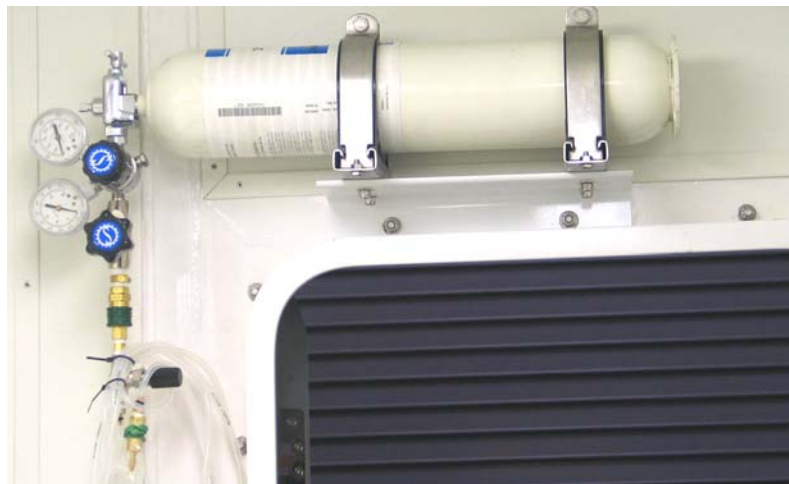
Figure 2-13. Calibration Sample Gas Cylinder
