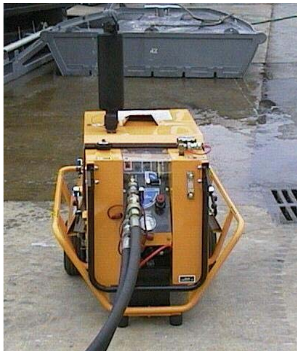
Mod 9 HPU Front View
