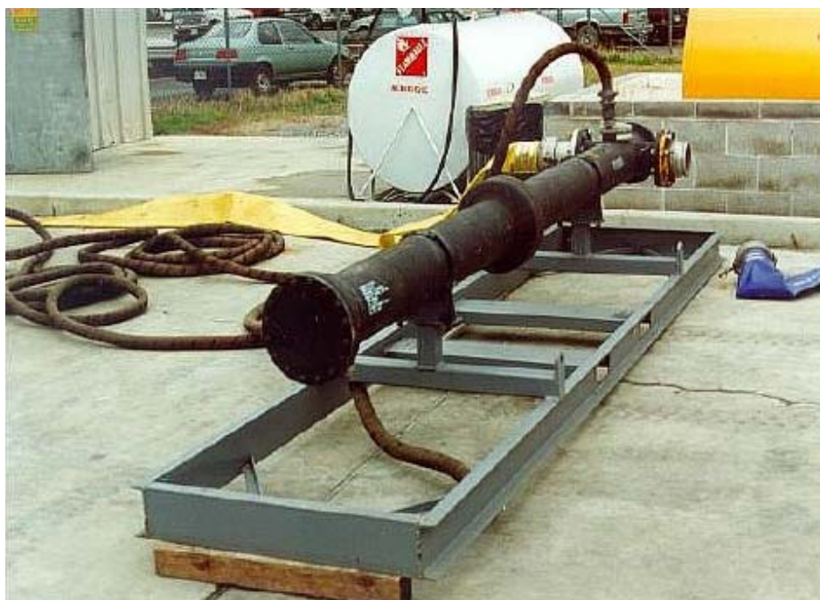
Oil/Water Separator External Heater SR0820
