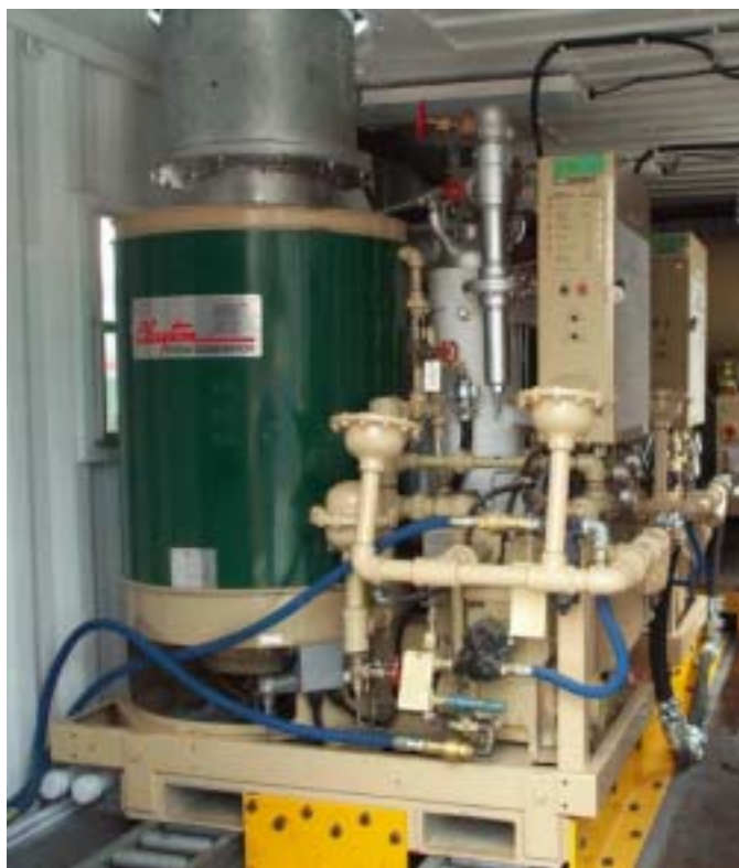
Steam Generator SG0010
