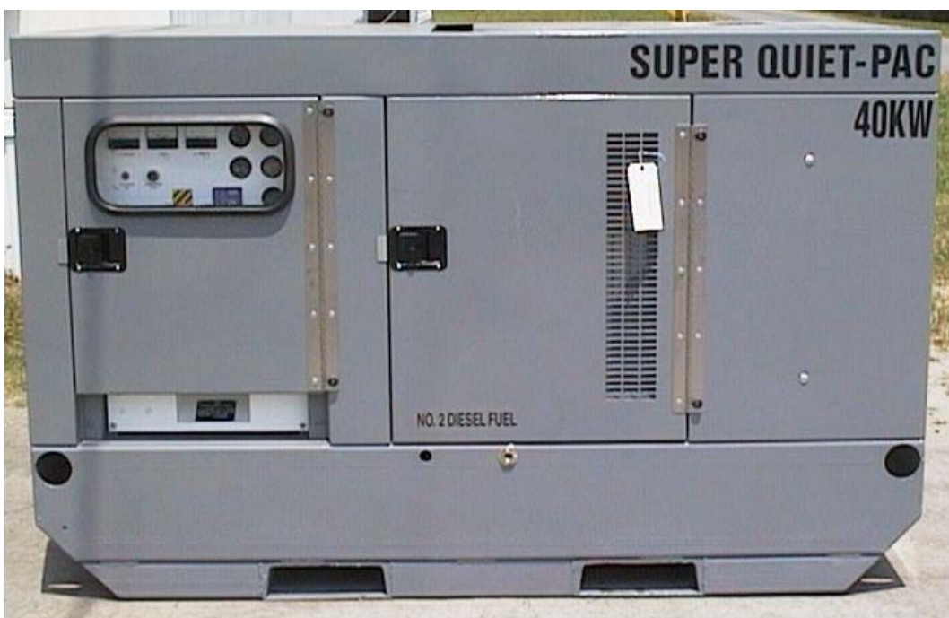
40-kW Diesel Generator GE0550
