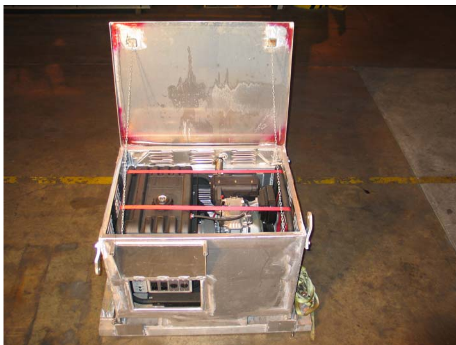
6.2-kW Diesel Generator GE0430
