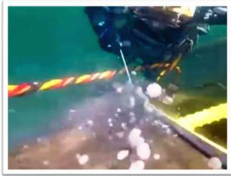
Fig. n° 10: Flammable bubble stream generated by a welding electrode (17).
