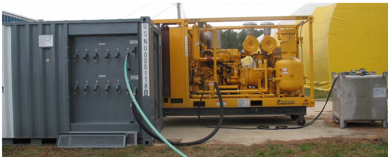
Overview of Submarine Salvage Air Compressor System S01300
