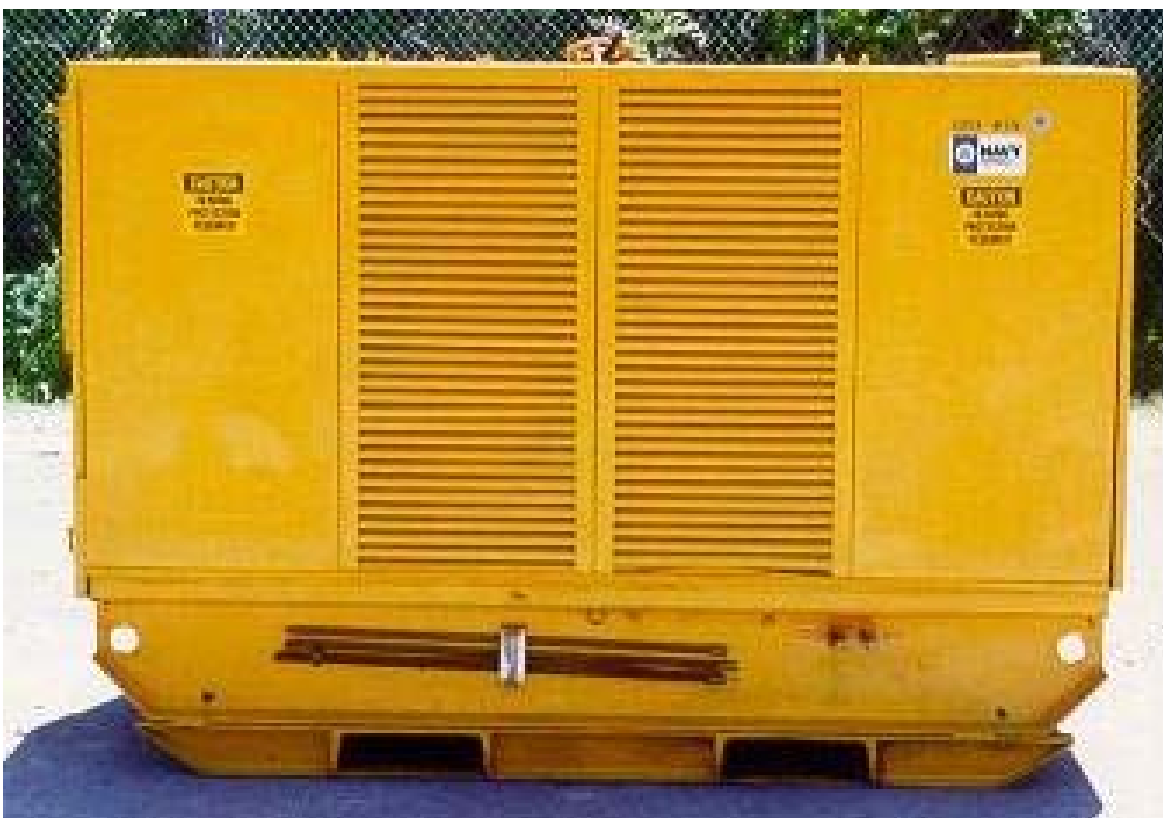
30-kW Diesel Generator GE0410
