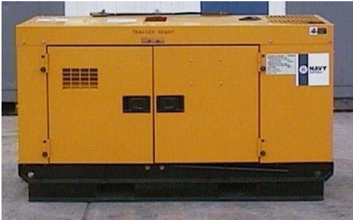
20-kW Diesel Generator GE0500
