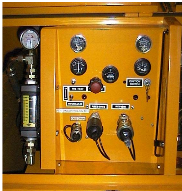
Mod 10 Hydraulic Power Unit Gauge Board
