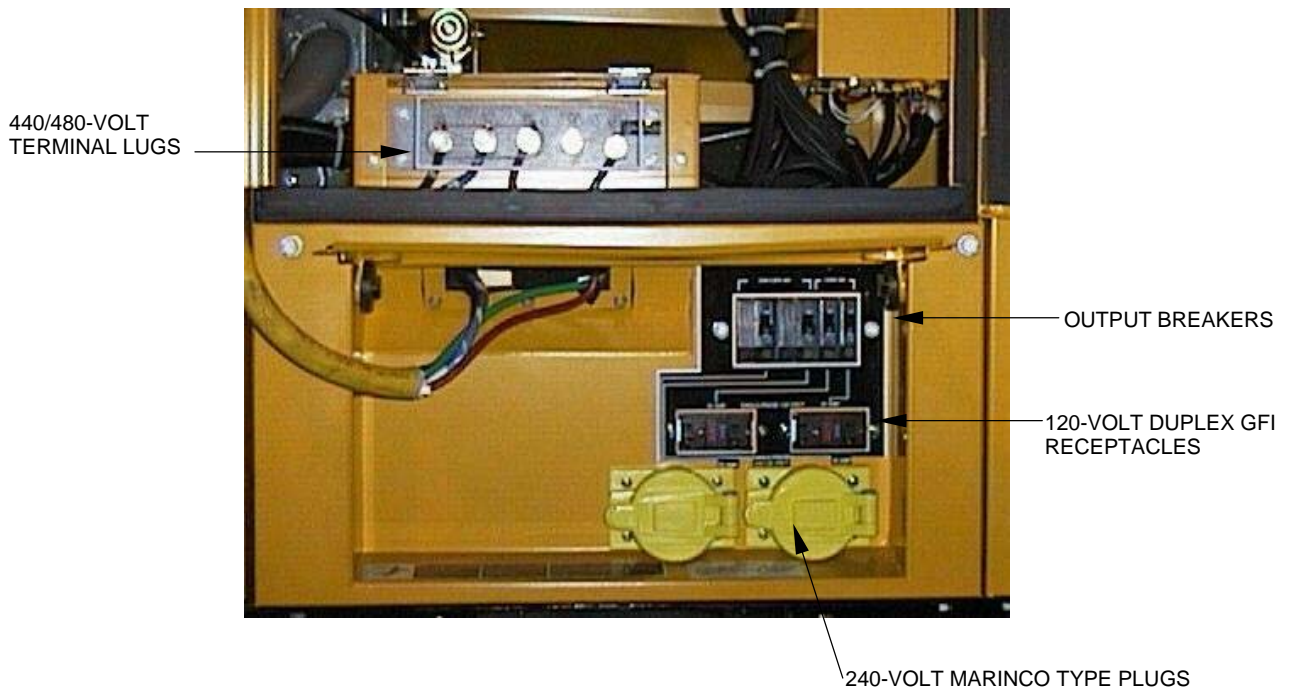
GE0500 Electrical Connections
