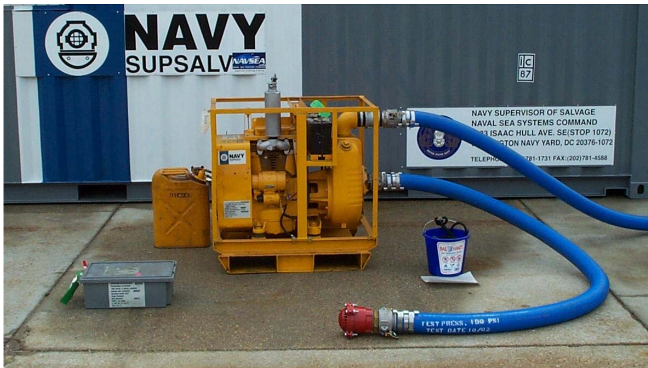
Configuration 1 – Diesel Driven Pump
