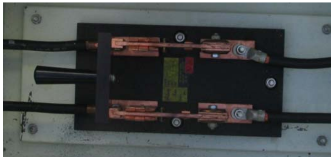
Switchbox Interior Showing Manual Switch
