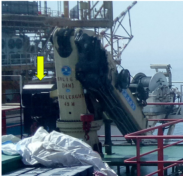
Control station in the open air
