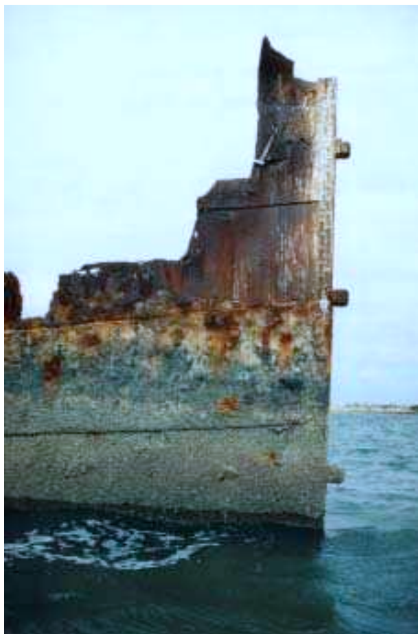
Figure 9.2 Stern of Moe at the Garden Island Ships' Graveyard (South Australia) showing missing rudder (Photo: Nathan Richards, 31/03/1997)
