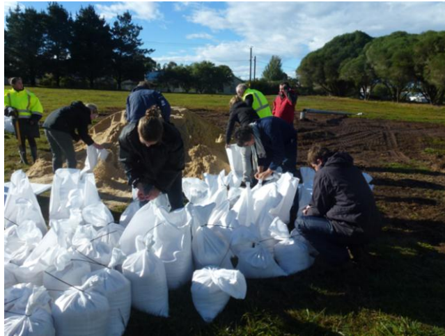
Figure 8. AHSP team filling sandbags to stabilise the site. Photo by J. Rodrigues.
