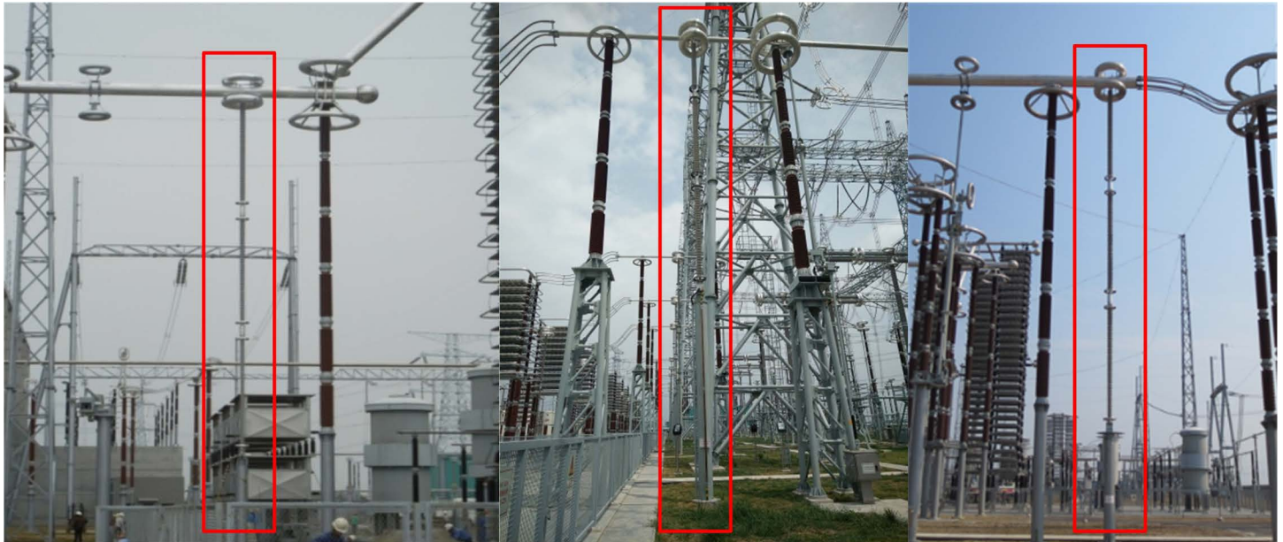
Fig 1. Field application of optical fiber current sensor.
