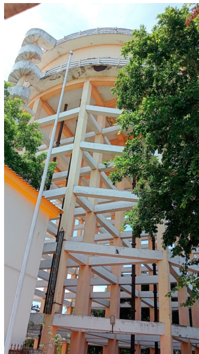
Figure 2. Overhead water tank located in Thirunallar, Karaikal, Puducherry, India.
