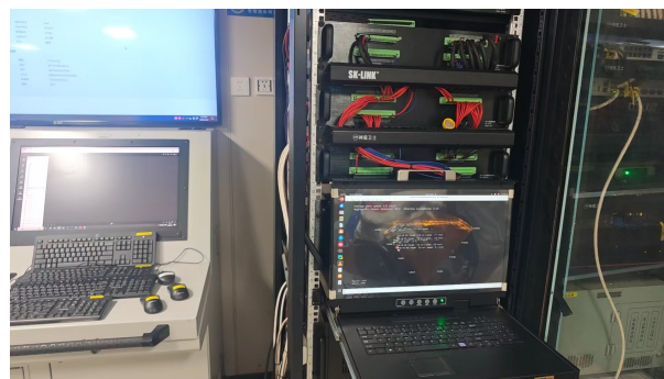
(b) Edge computing facility
